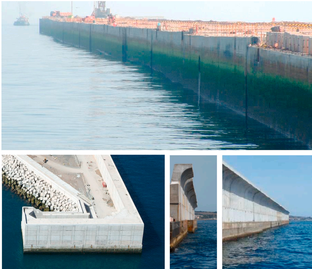
Fig. 1. Vertical caisson breakwater under construction (upper panel), corner section (lower-left panel), and recurved parapets (lower-mid and lower-right panels; courtesy M. Castellino).
