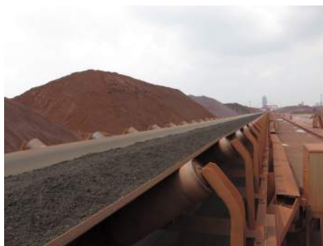
Figure 1.1: Part of a 1.5 km long belt conveyor system on a bulk terminal, figure courtesy of Rizhao Port Group Co., Ltd.
