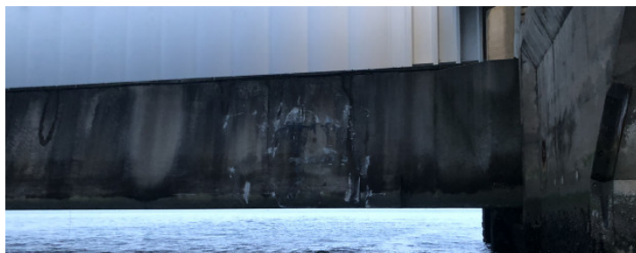
Figure 1.4: Damaged part of Oosterscheldekering after collision of Eemshorn ship [77]
