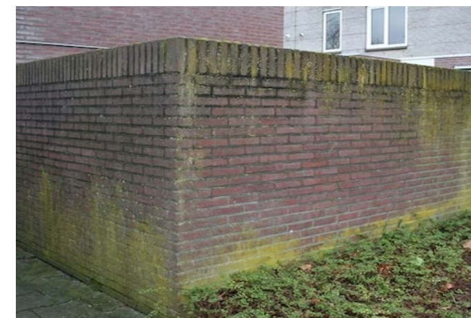
Figure 8.3. Example of a facade without predefined colonisation areas, where biological growth appears unintentional and is often perceived as deterioration (source: BN De Stem)
