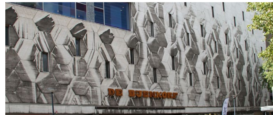
Figure 3.14. Facade of De Bijenkorf, Rotterdam, showing the accumulation of dirt due to the ribbed texture (Source: Sullivan, 2016)
