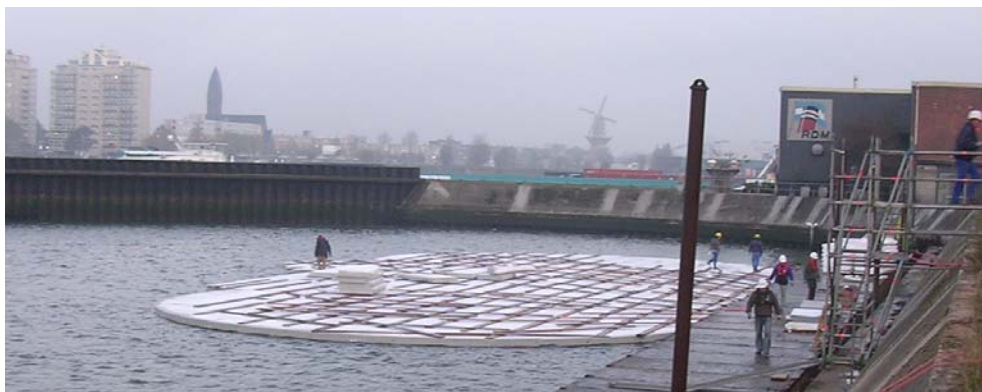
Figure 87: First layer of EPS of the floating pavilion, with planks on it
