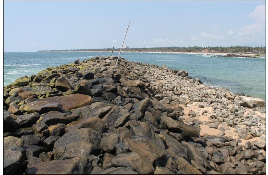
Figure R-23: Breakwater, displacement of armour stone
