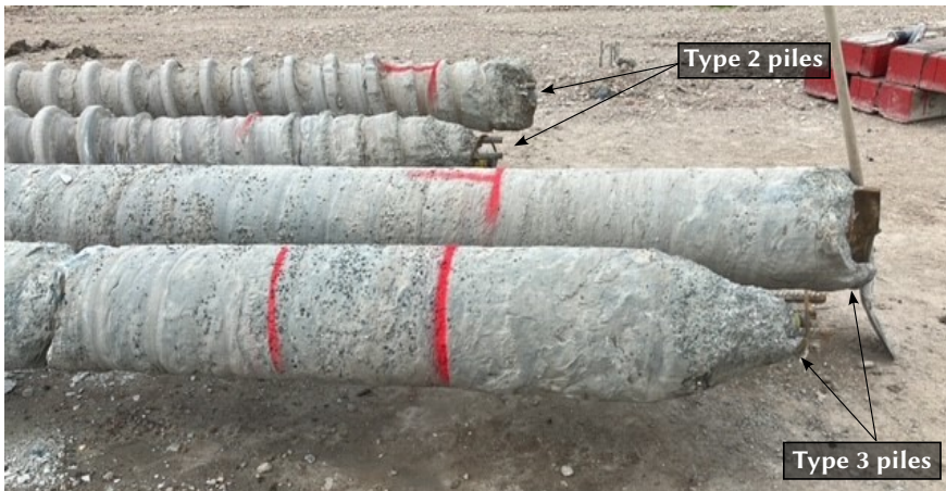
Figure 4.5: Base of four extracted screw displacement piles, all installed at the site.
