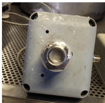
Figure 5.9: Blockage of the flow meter
