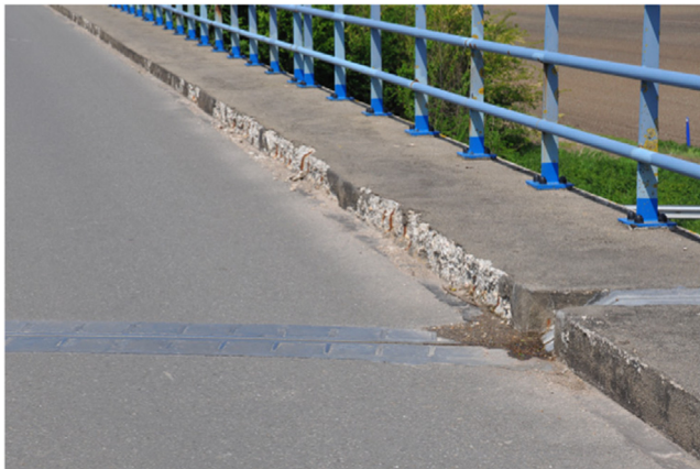
Figure 6.6 Concrete deterioration of the sidewalk.
