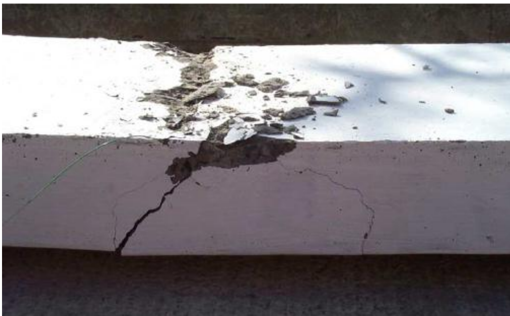
Figure 91 bending, and ultimately crushing, as failure mode for a laterally restrained reinforced concrete slabs (Taylor, Rankin, & D.J., 2001)
