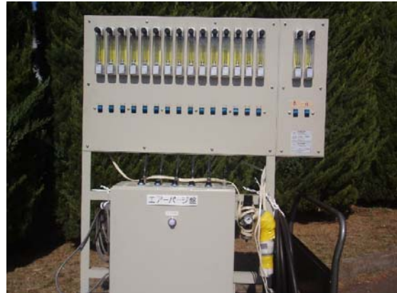
Figure 7. Flow Control Panel
