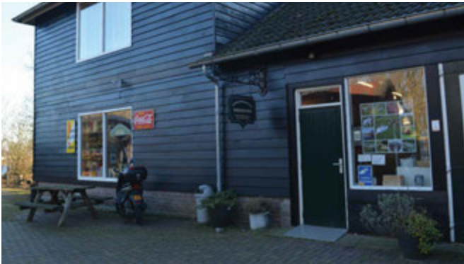
Entrance | needs improvement
