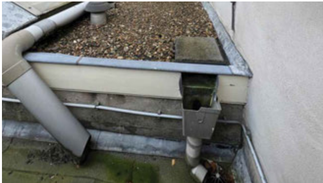
5 Down pipe system | urgent improvement needed
