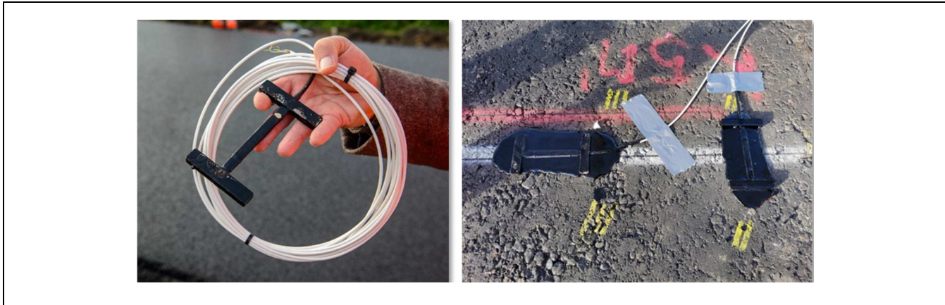
Figure 2. Strain gauge (left) and its installation at the top of the bottom layer (right).
