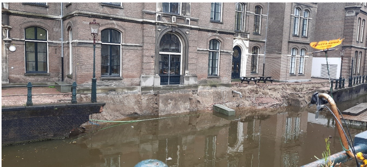
Figure 1.1: The collapsed Grimburgwal in Amsterdam [6]
