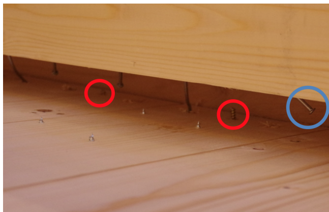
Figure 5-34: Failure of nails and screws at top joist
