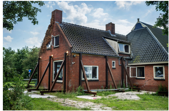
Figure 2-2: A temporarily strengthened house in Groningen [2]
