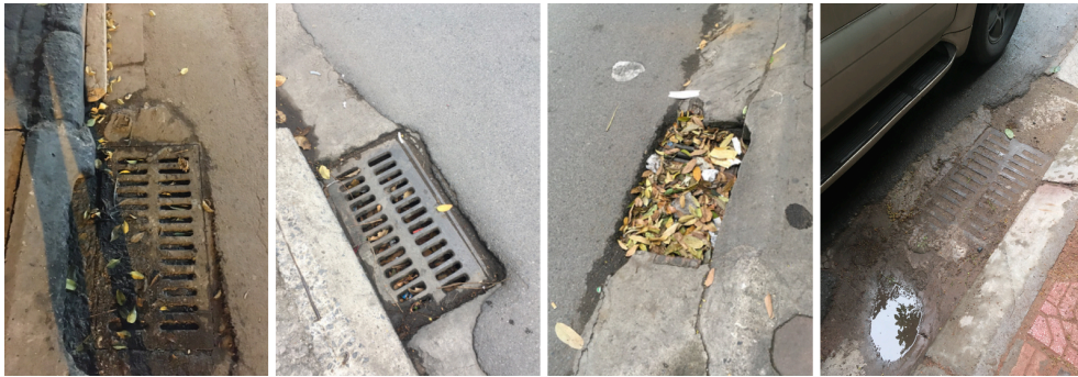
Figure B.4: Blocked drains due to a lack of maintenance
