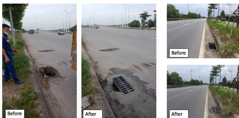
Figure B.3: Drains with stolen lids before and after repair work. Source: Hanoi's drainage company, pictures taken by Nguyen Trong Nam
