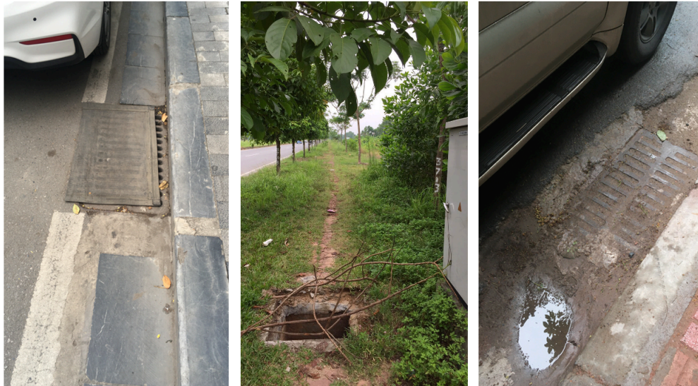
Figure 5.1: Observations from the site visit. Left: inhabitants placed a mat on a drain. Middle: stolen lid, leaving an entrance for large objects. Right: blocked drain due to lack of maintenance
