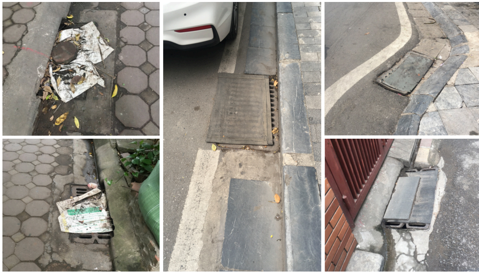
Figure B.5: Drains that are covered by mats or rubbish
