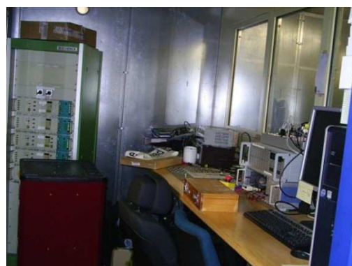
the control room
