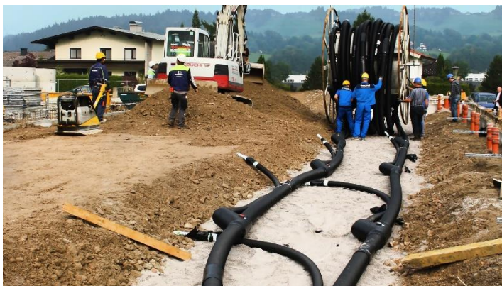
Figure 2-6 Installing PB pipes. The joints are on the big roll. Adapted from Thermaflex.
