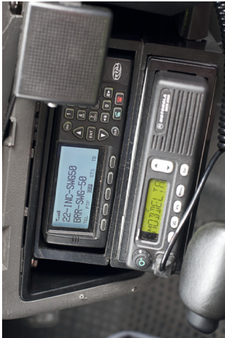
Figure 3.11. Digital TETRA mobile radio terminal and mobile analog radio terminal.
