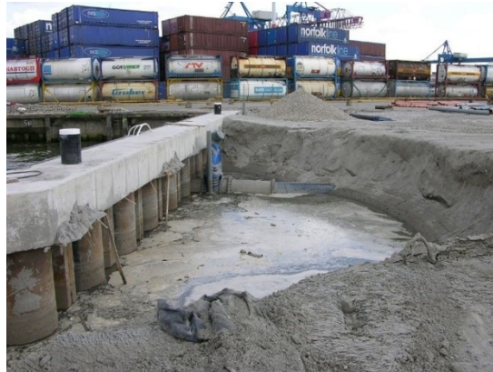
Figure 21. Hole due interlock opening in combi wall.
