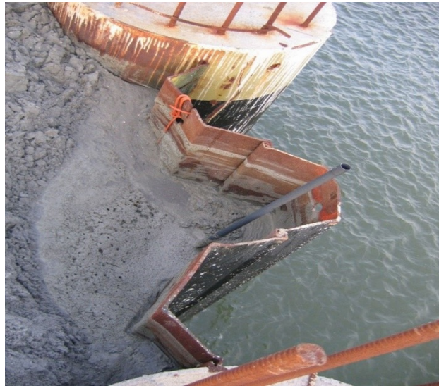
Figure 13. Failure due hydraulic fill behind quay wall.
