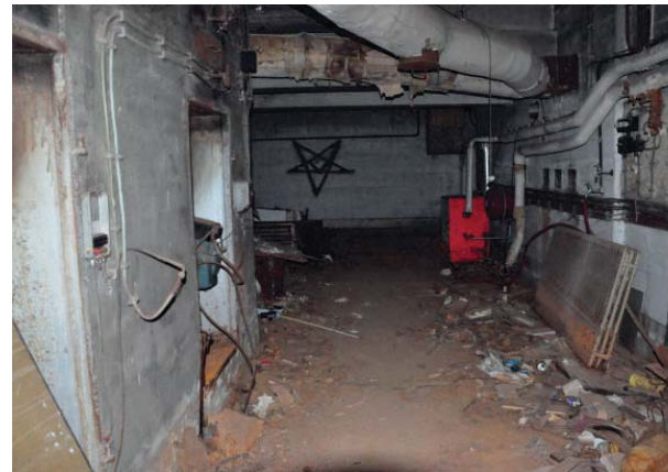
Figure 4.22: Basement with heating unit
