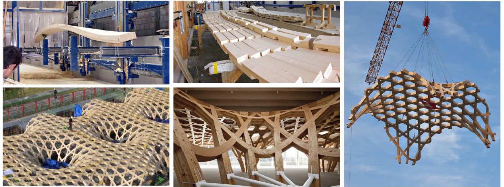
Bending of wooden elements (top left), Bent beams with grooves (top middle), Assembled roof (bottom left), Metal joint at supports (bottom middle), Assembly of a pre-fabricated roof segment (right) [Rondina, 2014]
