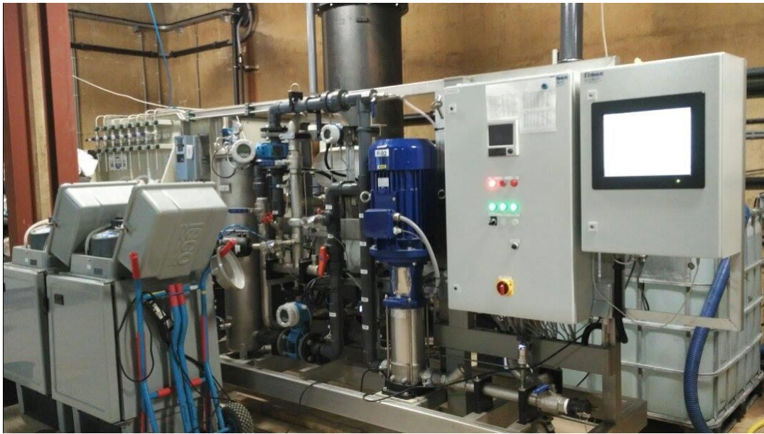
Figure 8: The installation that is used during the experiments in Kamerik.
