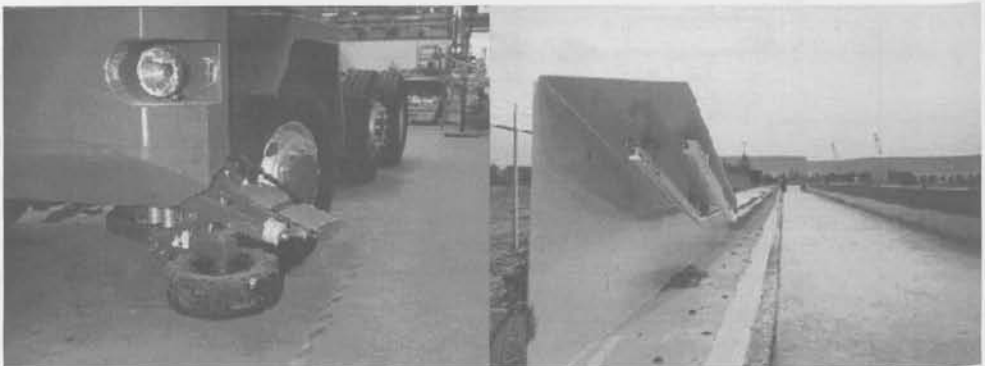
Figure 4. Current collector system.
