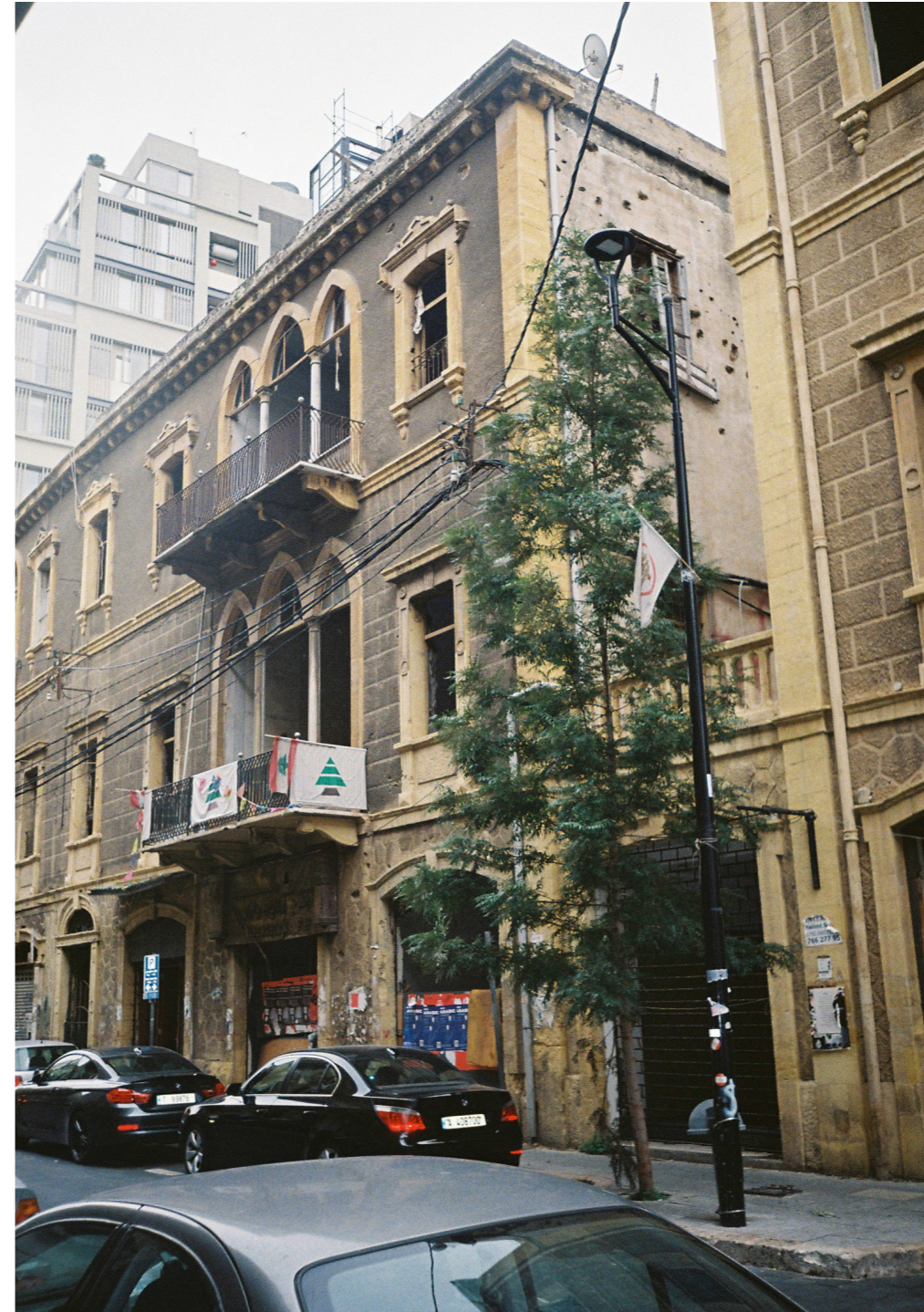
Figure 22: A heritage building close to the green line, with bullet holes penetrating the facade. The building is damaged by the blast. Personal photograph from case study.
