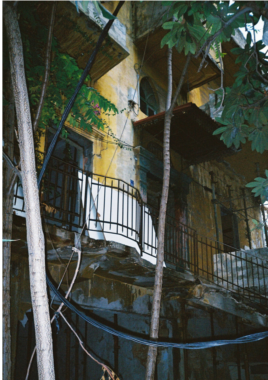
Figure 27: A damaged building in Gemmayzeh. Personal photograph from case study.
