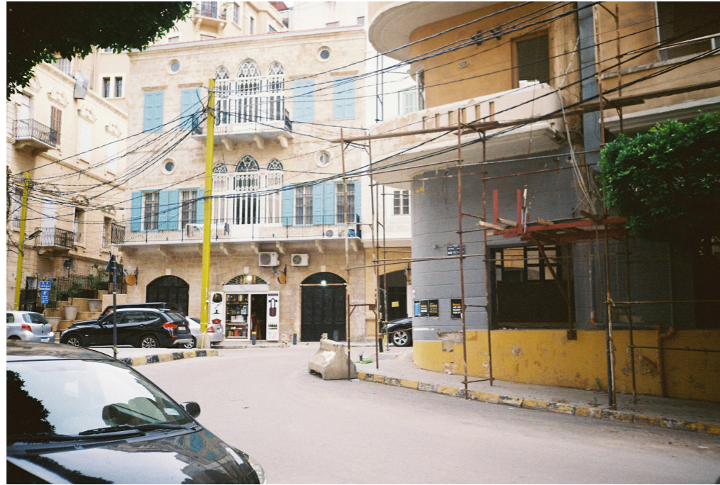
Figure 20: Construction site of damaged building on Armenia Street. Personal photograph from case study.
