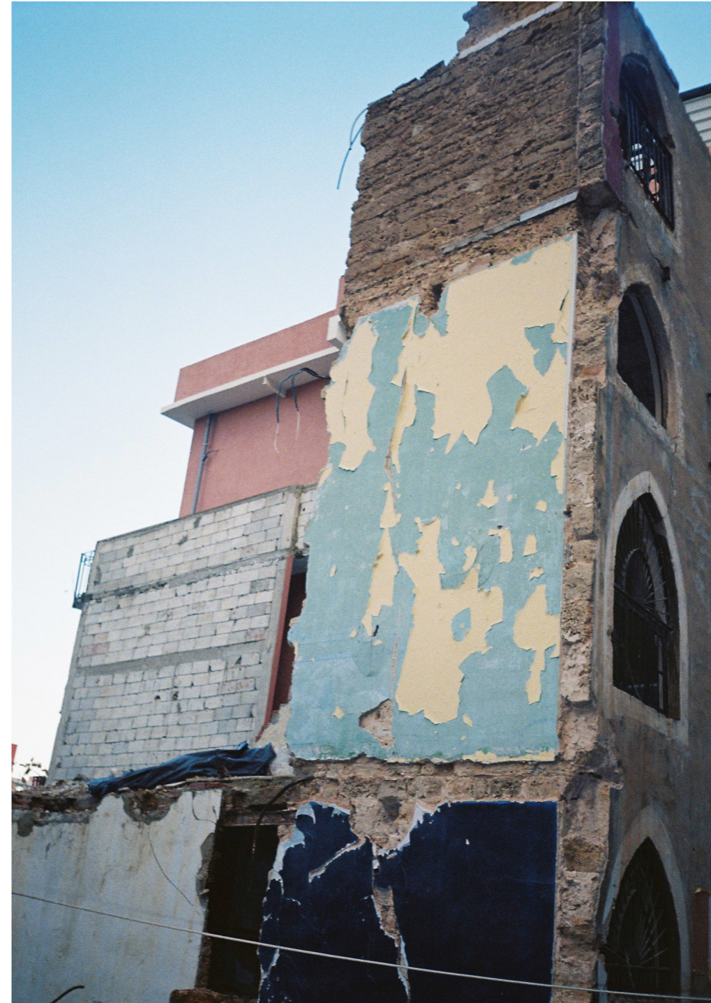
Figure 28: A completely collapsed building. The building collapsed due to it having an extra floor build on top of the original construction. A resident died at this spot. Personal photograph from case study.
