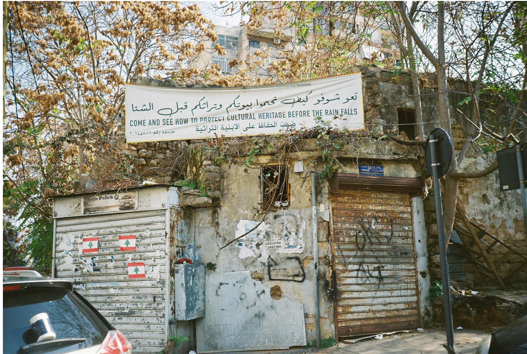
Figure 17: A call for the protection of heritage. Most heritage building roofs were blown off. The raining season would cause further damage to the structures. Therefore, one of the first actions was to cover heritage buildings. Private photograph, December 2022.
