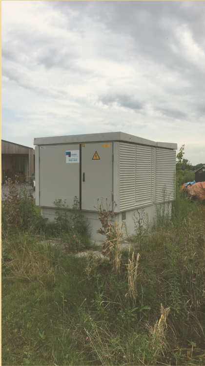
High-voltage electricity grid
