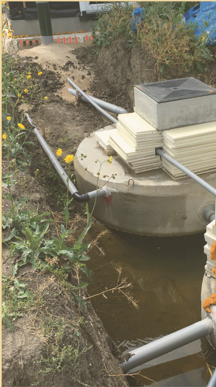
W2 Septic tank
