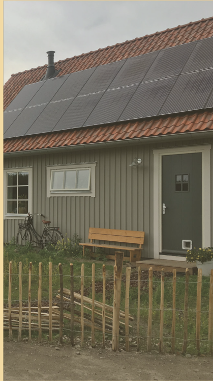
E1 Photovoltaic panels
