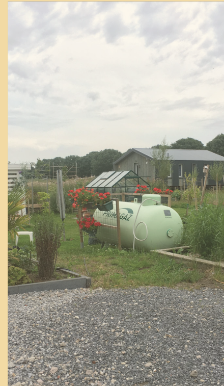
W3 Biogas Reactor
