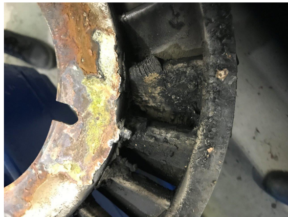
(b) Constipated nozzle-ring of Turbine section
