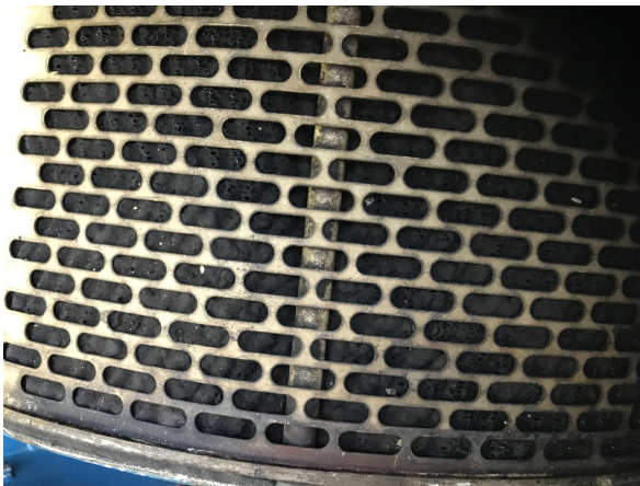
(a) Constipated inlet filter of Compressor section
