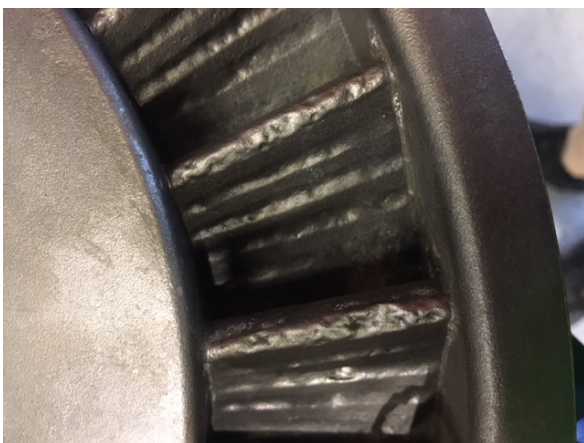
(a) Buckled and Penetrated nozzle ring of turbine section
