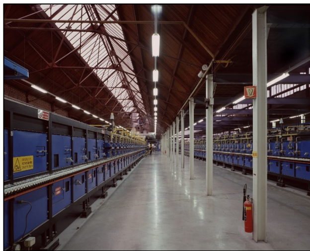
Figure 29. The outside of fast firing roller kilns (KNB, 2020a).
