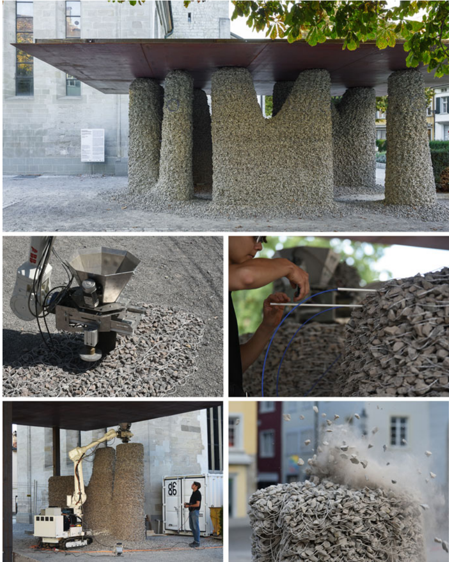
Fig. 9.1 (i) The Rock Print Pavilion is a full-scale robotically jammed structure composed of gravel aggregates and twine. The enabling technologies facilitating the on-site adaptive construction process include a custom robotic end-effector (ii) for extruding twine, depositing aggregates, and compacting layers, a structural health monitoring approach for the movement of the structure and the roof over time (iii), and mobility and localisation of the IF enabling the production of a larger structure on uneven ground (iv). The structure can be easily deconstructed with no material downgrading by removing the twine (v). (© Georg Aerni)
