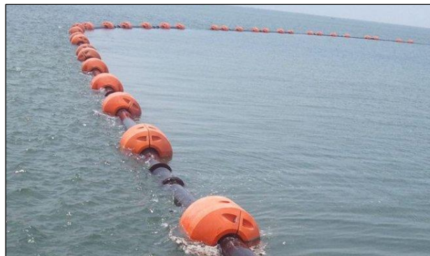
Figure 7-6 Small floating pipe line (ø 40 cm) in practice
