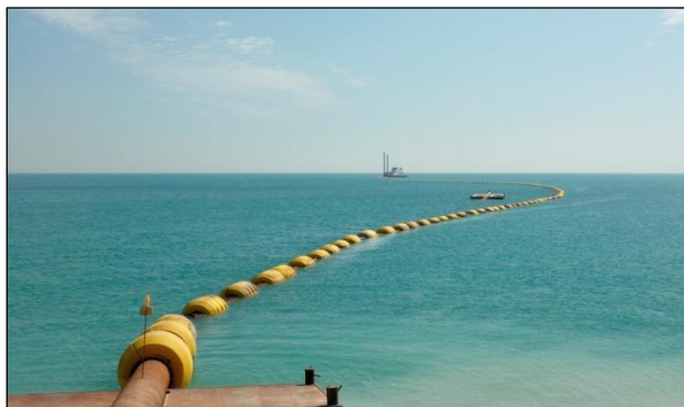
Figure 7-7 Cutter Suction Dredger connected with floating pipe line (ø 40 cm) towards the coast
