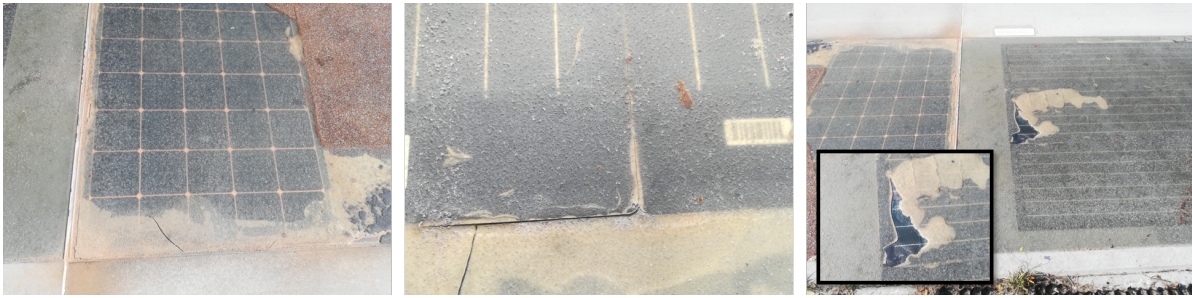
Figure 2.6: Soiling and delamination of the top layer occurred in the SolaRoad pilot site in Krommenie (July 2019)
