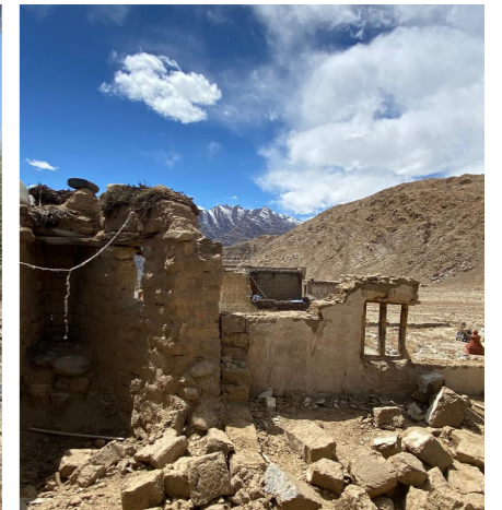
Architectural restoration still needed
