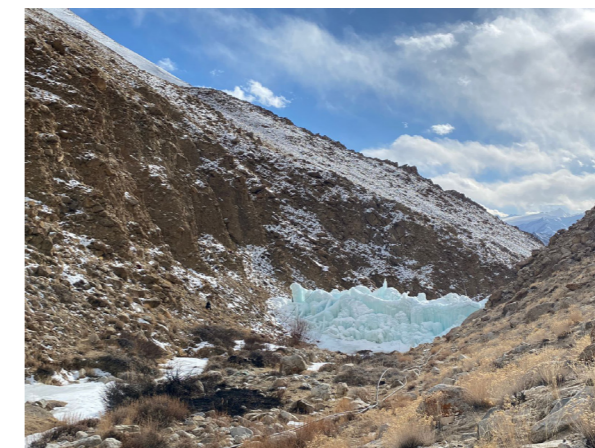
As ice accommodates, more piping can be added to increase the height of the structure.
