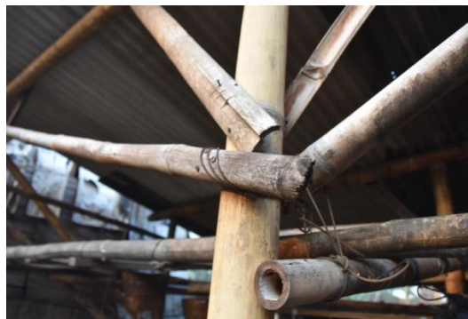
Figure 2. Poor Bamboo detailing and treatment causing splits and rot. Photograph taken by the author on 5 th November 2019.
