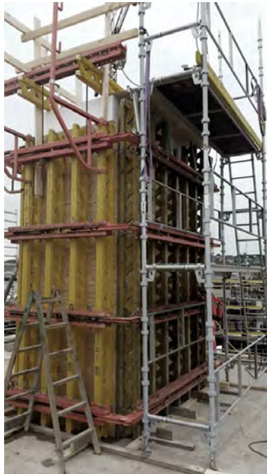
Figure 4.3: Onsite prefabrication using a standard, rectangular scaffolding for formwork support against bespoke EPS infills.
