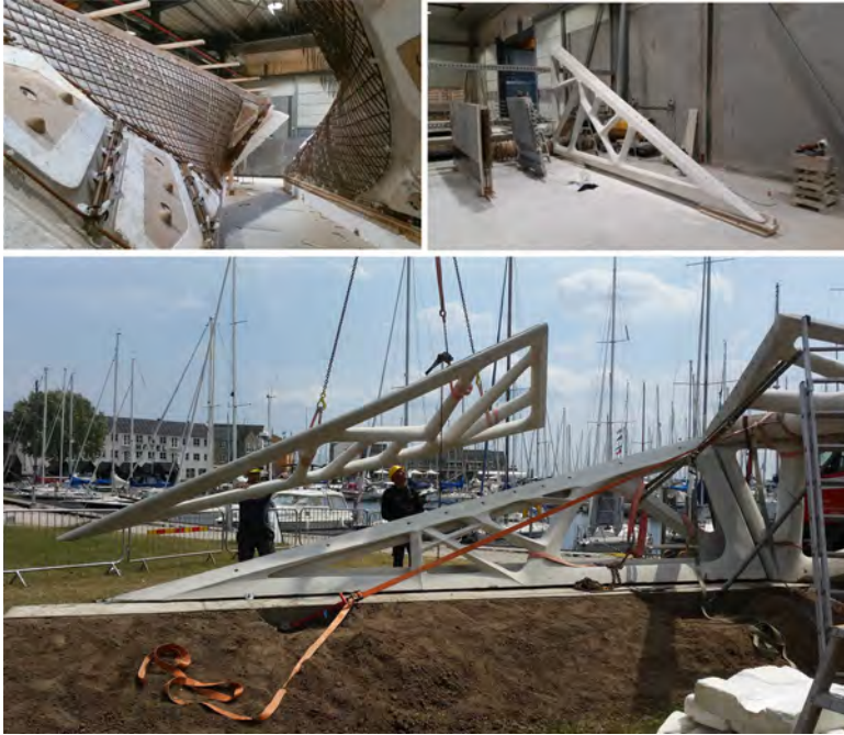
Figure 3.32: Reinforcement of element B1 (top, left) and element A1 after casting (top, right). Bottom: assembly of element A1 on A2, B1–B2
