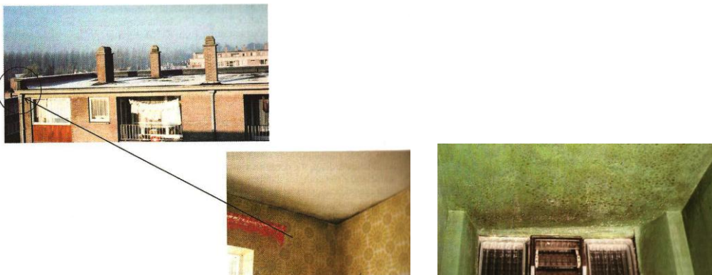
2.3.6 Internal condensation caused by thermal bridges, insufficient insulation and ventilation. (Hens, 2007)
