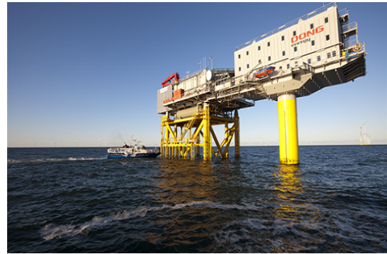
Figure 2.14: On the right is the accommodation platform next to the substation at the Horns Rev2 Wind farm (Energinet, 2015)
