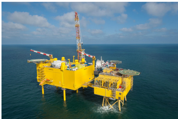
Figure 2.5: The BorWin alpha and beta substation platforms in the North Sea, adapted from (TenneT, n.d.)
