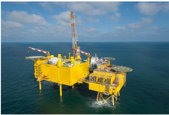
Figure 2.2: The BorWin alpha and beta substation platforms in the North Sea, adapted from (TenneT, n.d.)
