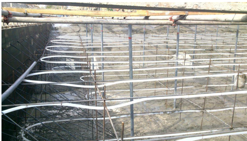
Figure 2-10 White cooling pipes are installed between the reinforcement to lower the maximum temperature (Kalhara, 2021)
