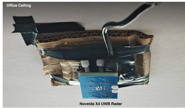
Figure 5.5: Image of the Novelda X4 radar installed on the ceiling.
