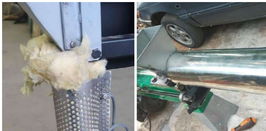
Figures 28 and 29: The insulation wool and sheet-metal insulators
