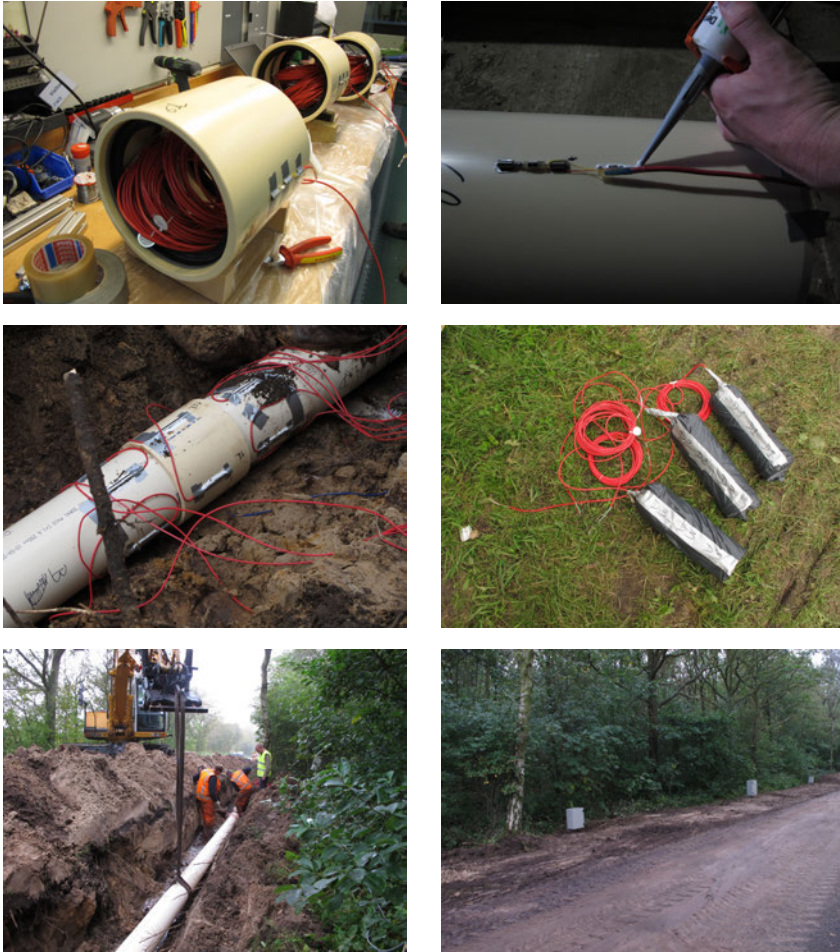
Figure 4.2: Photos taken during the installation of the sensors. Top left: the strain gauges fixed on the joints. Top right: a strain gauge being fixed on a pipe. Middle left: the dummy strain gauges inside sealed PVC canisters. Middle right: the installation of the pipe. Bottom left: the strain gauges fixed to a joint and two pipes. Bottom right: following the installation, the three cabinets are visible above ground.
