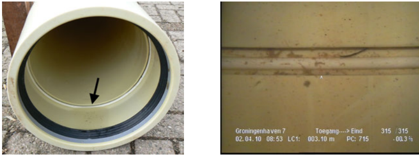
Figure 3.1: Left: image of the interior of a 315 mm PVC joint. The gap is signaled with an arrow. Right: underwater image of the interior of the same PVC joint obtained with CCTV. Please note the difference between this joint and the one presented in Figure 2.2: in this situation the ring separating both joints (white) was molded with the joint and is not a stand-alone piece.
