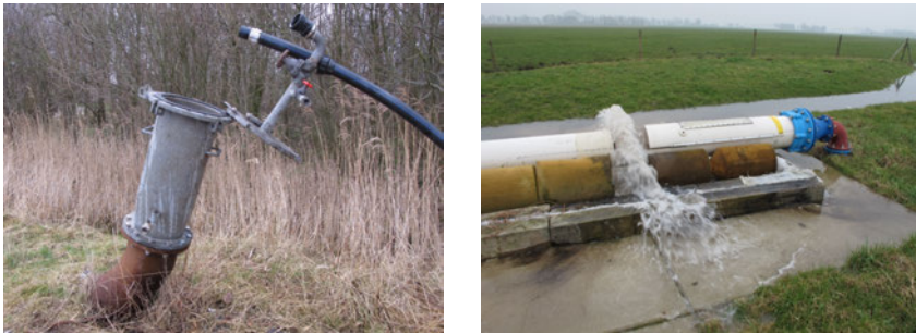
Figure 3.11: Entry point with flange and hose (left). Exit point with sliding door above ground level (right).
