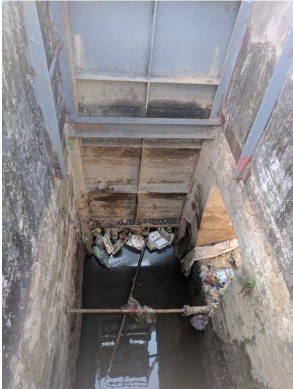
(a) The inside of the FGS under low water level conditions. It could be observed that even without a rainfall event flushing a lot of waste to the gate structure there is a significant amount that is stuck within the structure. Moreover, the observation also shows a pipe or cable that runned through the structure. This could potentially increase the probability that waste gets stuck. Picture taken February 8, 2017.
