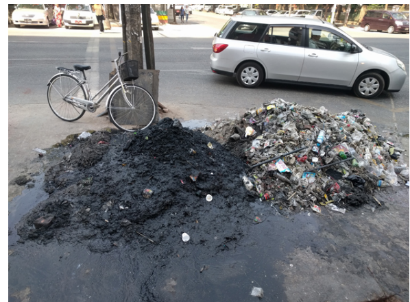
(b) This was an example of the waste and deposits that were removed from a culvert that was cleaned on a monthly basis (outside of Latha though). The amount of waste was from one half of the culvert and the cleaning operation was still under way when the photo was taken. Picture taken on March 15, 2017.
