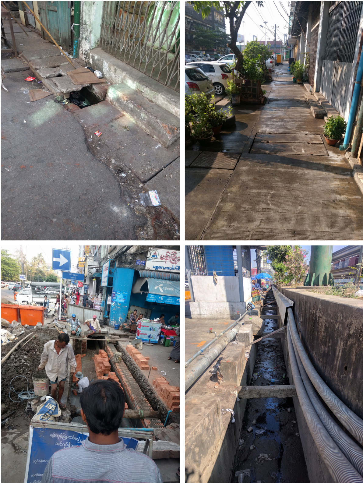
Figure C.10: The drains canal drains had different types of concrete slabs that cover them off (top left, top right). The smaller slabs were more often partially broken or missing, as opposed to the larger slabs. The drains and culvert were made from a combination of concrete and bricks (bottom left, picture taken on 39 th Street). Some of the drains were even without a cover, as for example the drains along the south side of strand road (bottom right). Data obtained by field observations between 01-03-2017 and 30-03-2017.
