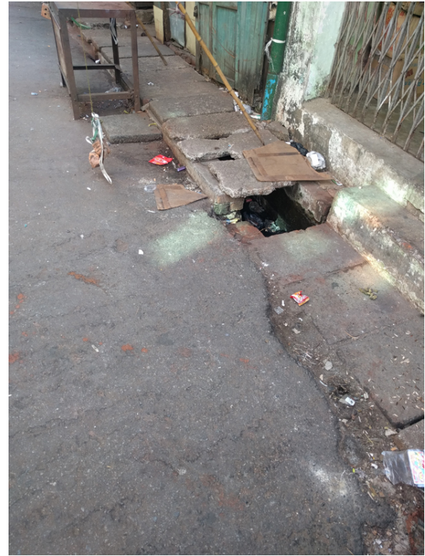
(b) For a lot of locations the maintenance state of the drains was not 100%. Such cracks and openings were often used as a place to dispose waste, as could be observed by the amount of waste in the drain around and under the opening. Picture taken on March 5, 2017.
