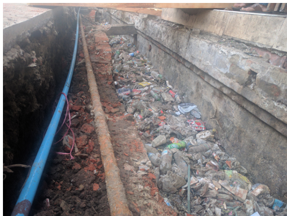
(a) A drain that was broken open for reconstruction provided a nice insight in the amount of waste that can be present in a drain. The drain was not situated in Latha, but this was not out of the ordinary for the drains in the busiest streets of Latha. Picture taken on January 8, 2017.
