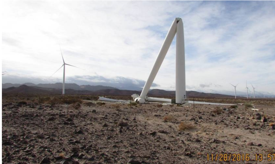
Figure 2-8: A buckled wind turbine, caused by local buckling of the tower[Unknown].
