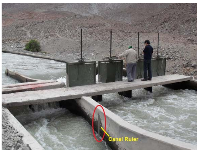
Picture A6-1 Division Structures and Canal Ruler at the Beginning Of Lateral 1
