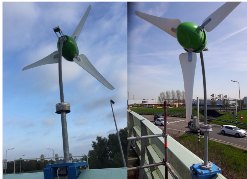
Figure 1. Micro wind turbine integrated on top of the noise barrier.
