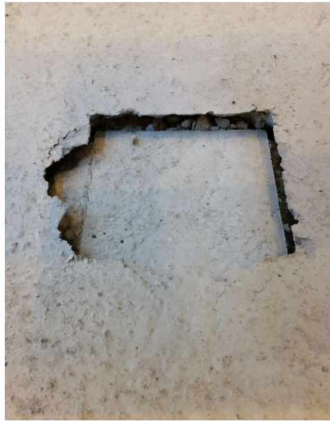
Figure 7.53: The loading plate punched through the top layer of the concrete.
