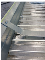
(a) A connector preventing the longitudinal sides from bending outwards due to the weight of the wet concrete
