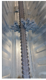
(a) A picture of a reinforcement bar placed in the rib of a deep steel deck
