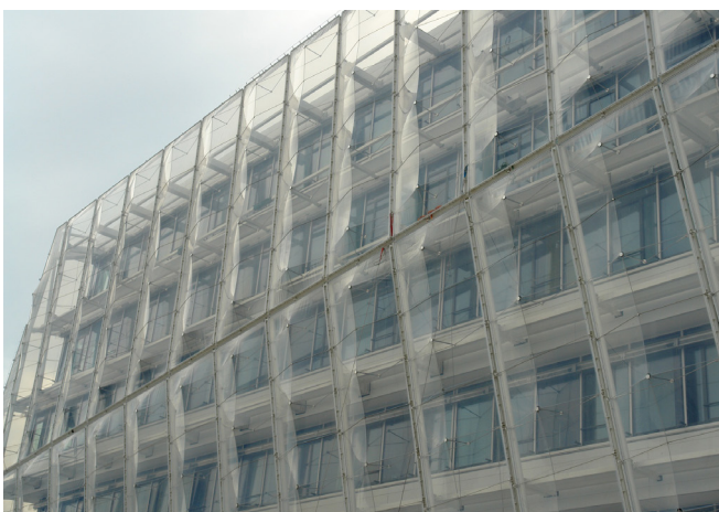
Figure 111: ETFE Facade at the Unilever Building in Hamburg. [source: ETFE facade Unilever building, Hamburg. (n.d.). Retrieved from https://www.tensinet.com/index.php/about/members-of-tensinet?view=project&id=4456 ]
