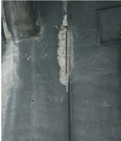
1 Spalling of concrete
