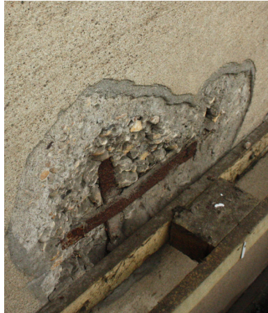
2 Corrosion of the reinforcement
