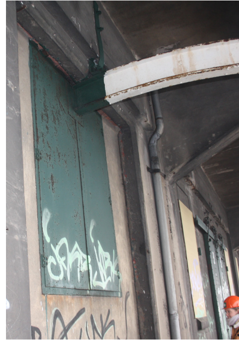
Image 3 - Rail through doors
