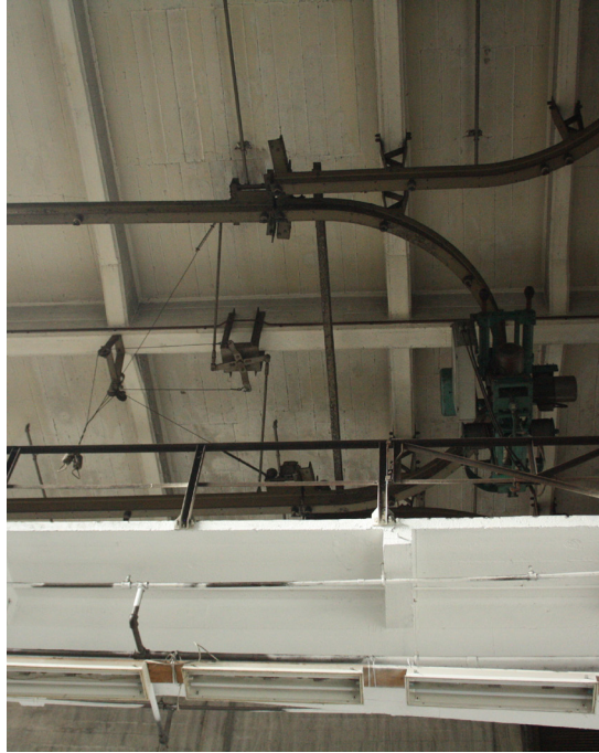
Image 2 - Rail changing system and operating cables
