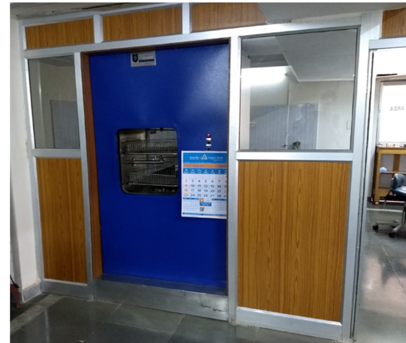
Fig 5.2.2 Unused washer-disinfector in hospital A
