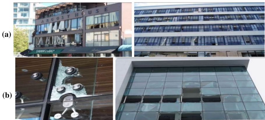
Fig. 1 Damage observed in the 22nd February 2011 Christchurch earthquake to a traditional glazed curtain walls and b Point Fixed Glass Facade Systems, Baird et al. (2011a)
