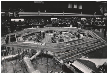
A trading pit under construction during the 1987 expansion of Chicago Mercantile Exchange. The trading pit was elevated to contain air ducts, which cooled of sweaty traders. Source: tradingpitblog.com/2012/02/depth-of-mar- ket.html
